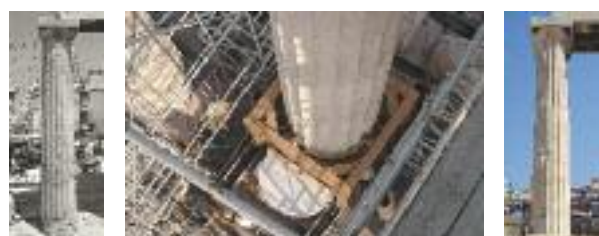
The fifth column from the east on the south side before, during and after the restoration.
