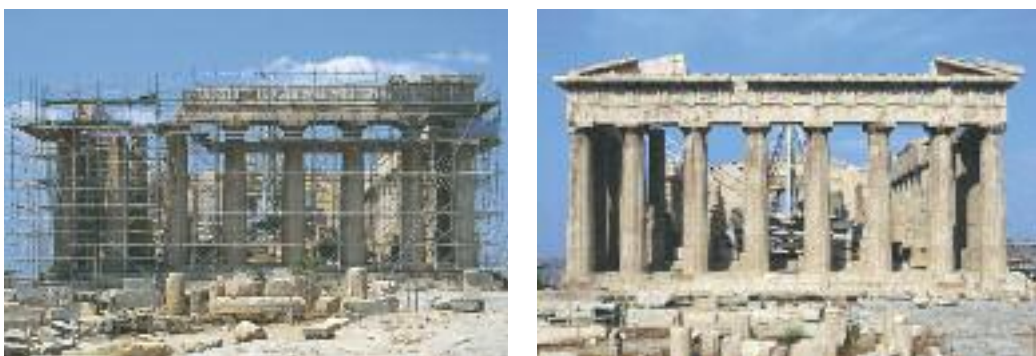
The east façade of the Parthenon during and after completion of restoration.
