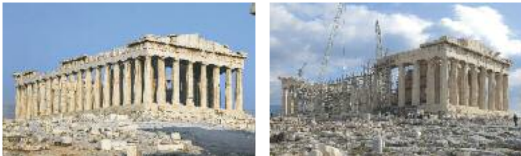
View of the northwest side of the temple before and during the works.
